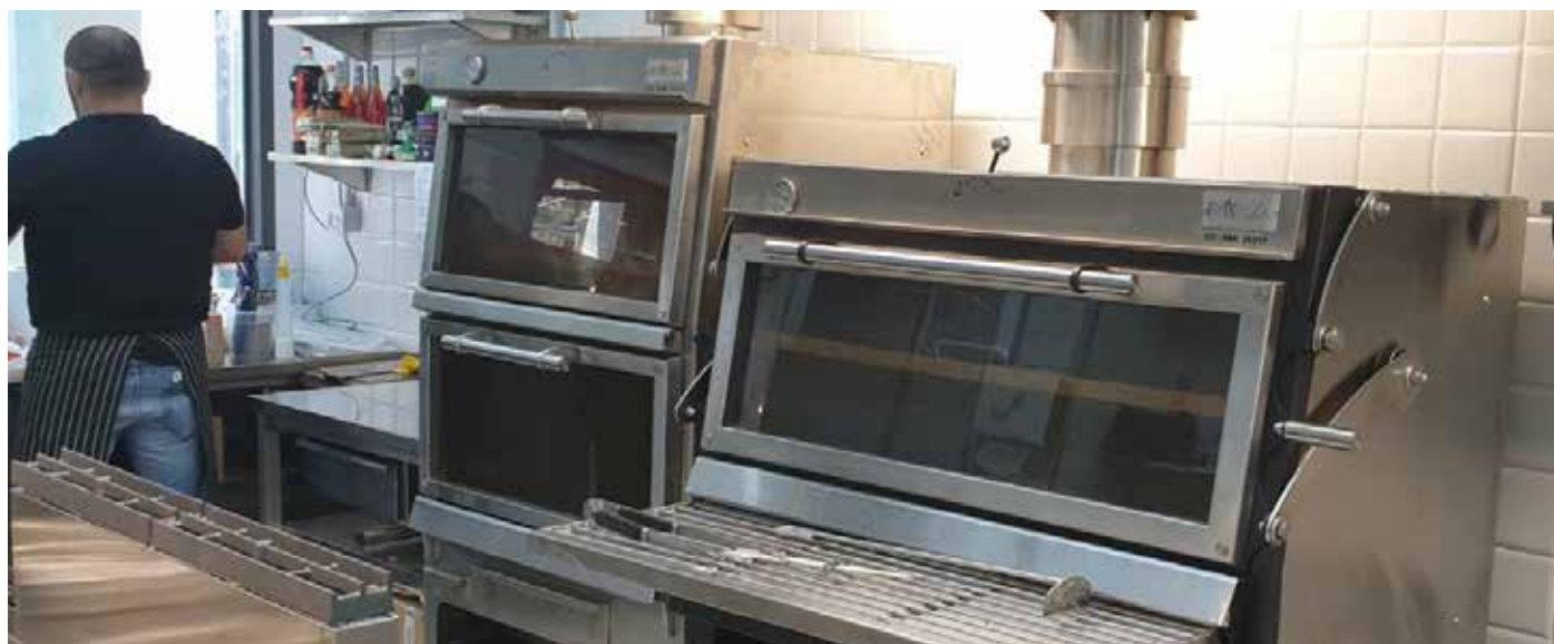
Ara Bracis Restaurant kitchen detail in Rome
